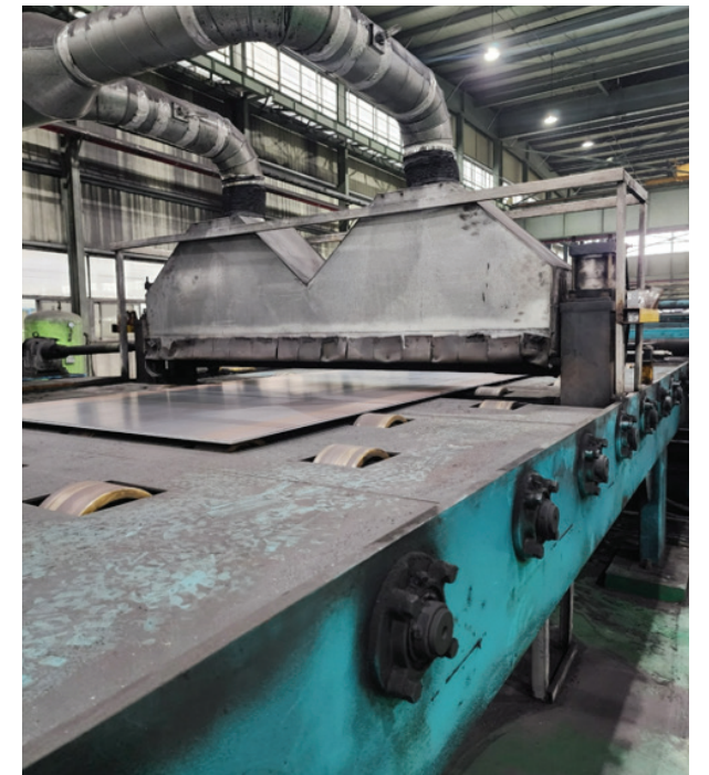
Dust collection facility at SeAH L&S's Dangjin Plant
